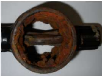
badly scaled valve Feb 2009
