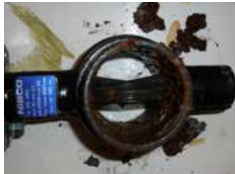
11 weeks after Aqua-Rex was installed
