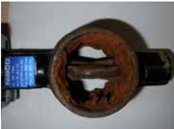
badly scaled valve Feb 2009
